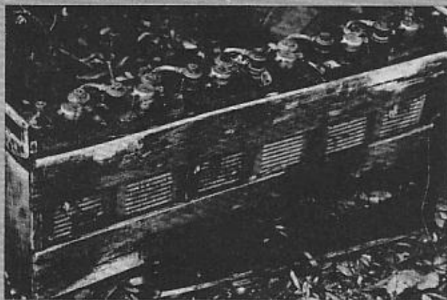
A battery of six Edison cells as collected on a salvage expedition. Most of the cells are good, but the original wooden rack is in bad shape. These are A-8 cells, originally rated at around 220 Ah each.
