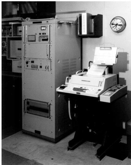
FIGURE 13.4. Photograph of below-deck equipment (BDE) installed in a ship cabin. (Courtesy of Anritsu.)
