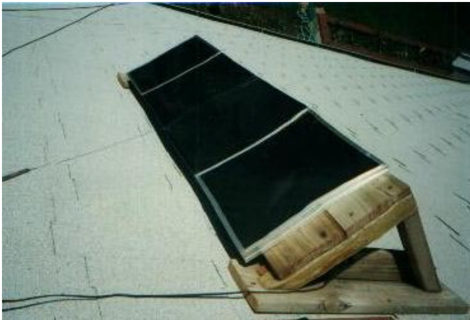
Solar panel on the roof
