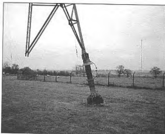
Fig 1.13: The entire mast is insulated from ground. Note the spark gap across the insulator.
